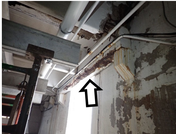
Photo 3 – Deteriorated Concrete Beam
