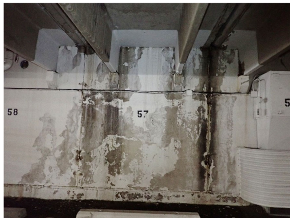
Photo 2 – Deteriorated Precast Wall Panel
