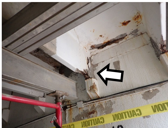
Photo 4 – Deteriorated Precast Double-Tee
